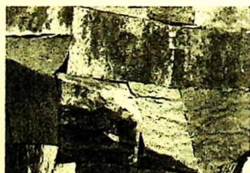
Crumbling Wall, 2000 (detail)
